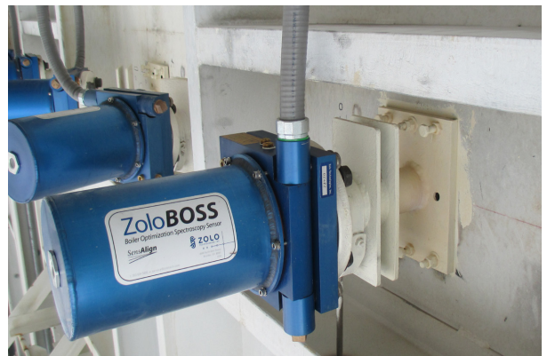
ZoloSCAN SensAlign heads mounted on the side of the furnace wall (above). The heads automatically realign as necessary to ensure optimum power transmission.
